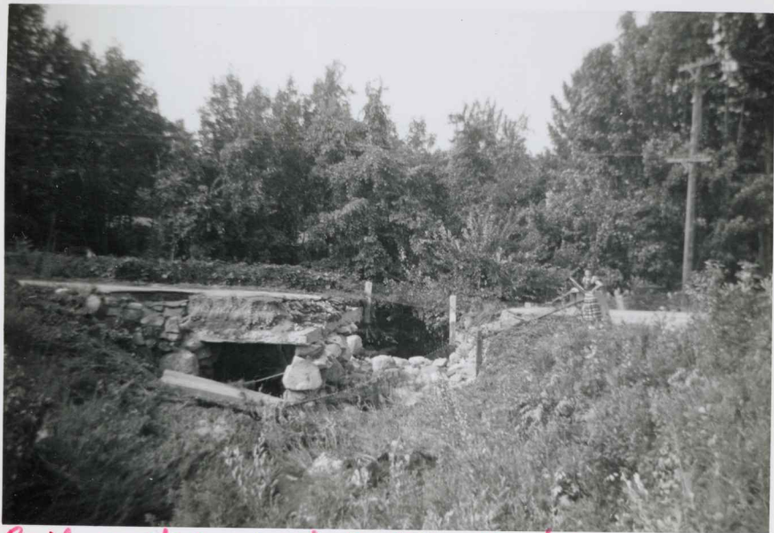
Bridge out in Wetherington. -flood 1955
