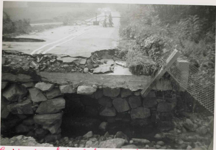
Bridge & Road Washed out by flood of 1955
