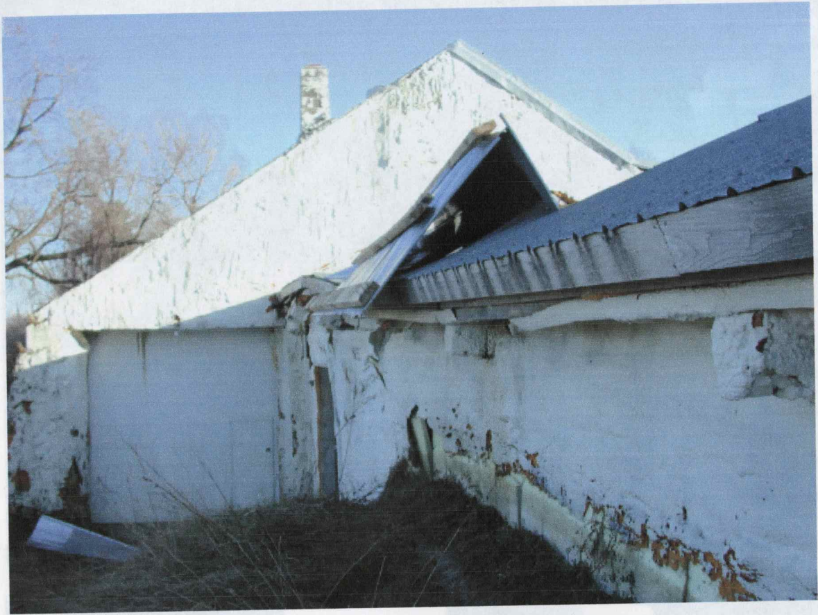
1 COND OF HEALTH INSPECTION - Friday April 16, 2004 - 5:30 PM Albert Property - Hummingbird Road, Worthington, MA
